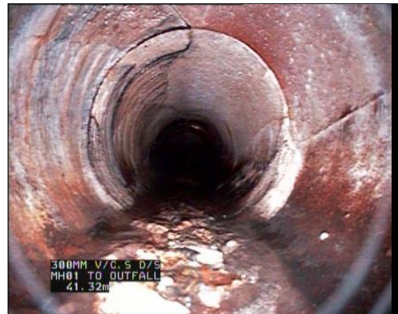
Photo: 12_12_129_A.jpg, 00:07:12 41.3m, Cracks, multiple, from 8 to 4 o'clock
