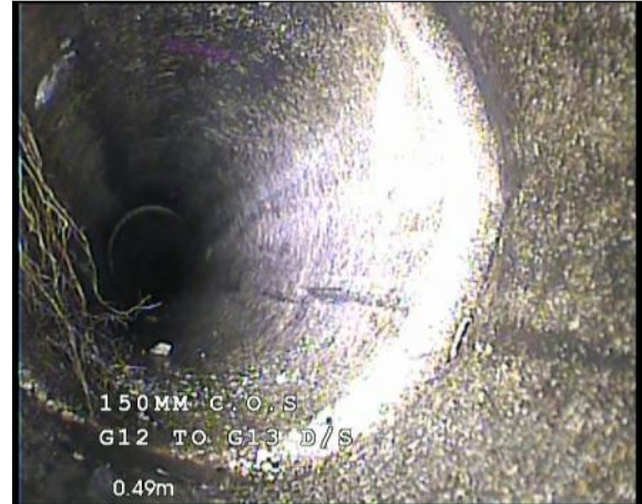
Photo: 16_16_218_A.jpg, 00:00:17 0.5m, Roots, fine at joint, Start
