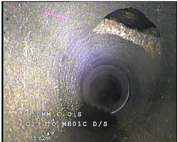
Photo: 22_22_254_A.jpg, 00:02:21 15.6m, Hole in drain/sewer, from 11 to 1 o'clock Remarks: POSSIBLE POOR REPAIR
