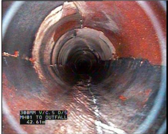
Photo: 12_12_131_A.jpg, 00:07:32 42.6m, Fracture, multiple, from 12 to 12 o'clock, Start
