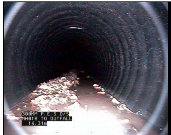
Photo: 25_25_278_A.jpg, 00:02:15 14.3m, Settled deposits, fine, 10% cross-sectional area loss, Start
