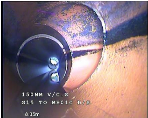
Photo: 23_23_265_A.jpg, 00:01:23 8.3m, Junction, at 3 o'clock, diameter 150mm
