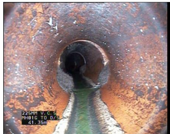
Photo: 33_33_385_A.jpg, 00:08:44 30m, Roots, mass at joint, 10% cross-sectional area loss, Start
