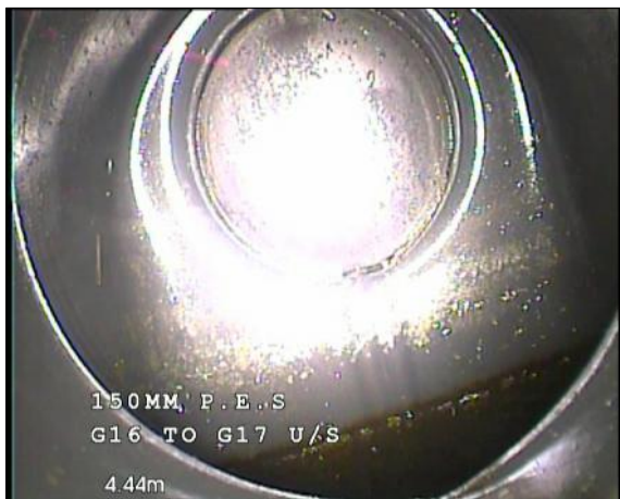
Photo: 18_18_231_A.jpg, 00:00:45 4.4m, Finish node type, gully reference number: G17 Remarks: TRAPPED GULLY 17
