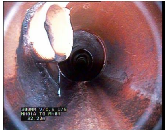
Photo: 11_11_113_A.jpg, 00:05:24 32.2m, Survey abandoned Remarks: UNABLE TO PASS INTRUDING CONNECTION
