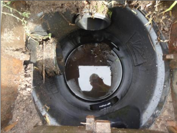
Photo: DSC02063.JPG 0m, Start node type, gully, reference number : G16 Remarks: GULLY 16
