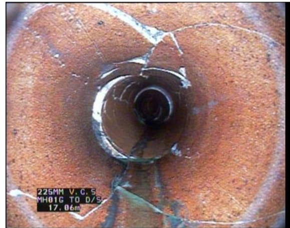
Photo: 33_33_377_A.jpg, 00:02:57 17m, Fracture, multiple, from 12 to 12 o'clock
