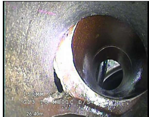
Photo: 22_22_262_A.jpg, 00:04:08 26.4m, Survey abandoned Remarks: UNABLE TO PASS POOR JOINT. MH01C IN VIEW
