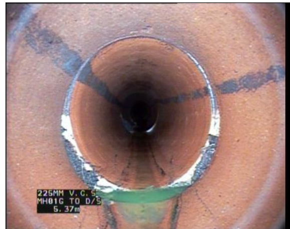
Photo: 33_33_371_A.jpg, 00:00:57 5.3m, Joint displaced, medium
