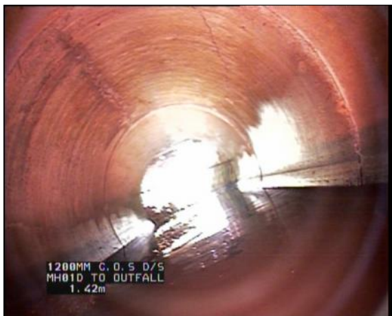
Photo: 27_27_297_A.jpg, 00:00:24 1.4m, Crack, longitudinal, at 1 o'clock
