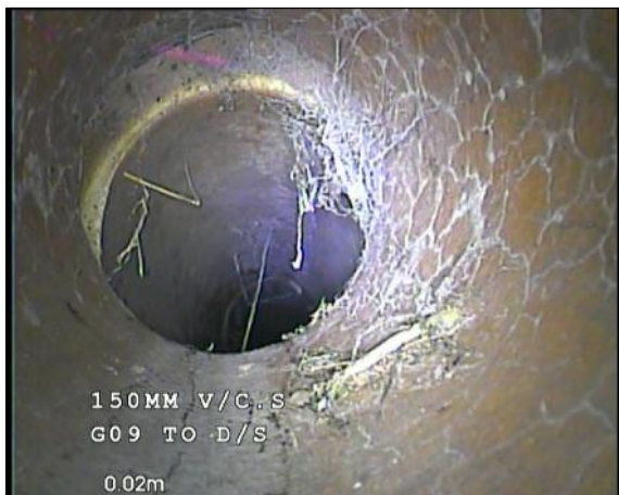
Photo: 9_9_93_A.jpg, 00:00:14 0.3m, Joint displaced, medium, Start
