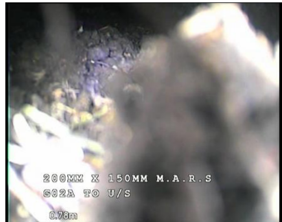
Photo: 31_31_338_A.jpg, 00:00:35 0.8m, Survey abandoned Remarks: UNABLE TO PASS HEAVY SILT
