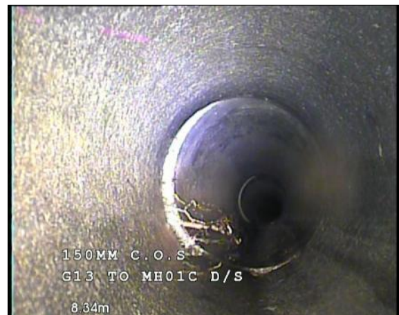
Photo: 22_22_246_A.jpg, 00:01:14 8.3m, Roots, fine at joint
