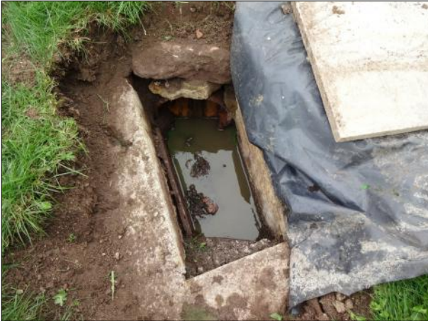
Photo: DSC02162.JPG 0m, Start node type, manhole, reference number : 01G Remarks: TRACED & EXPOSED MH01G
