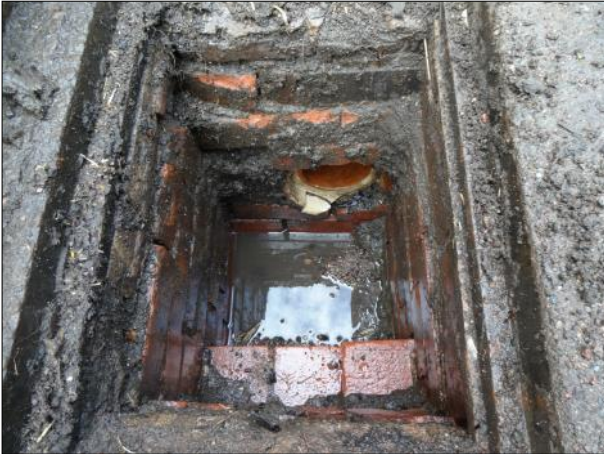
Photo: DSC02033.JPG 0m, Start node type, gully, reference number : G06 Remarks: GULLY 06
