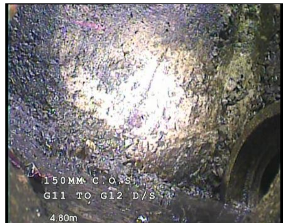
Photo: 15_15_215_A.jpg, 00:00:55 4.8m, Finish node type, gully reference number: G12 Remarks: GULLY 12
