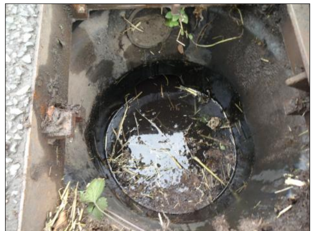
Photo: DSC02062.JPG, 00:00:45 4.4m, General photograph taken at this point Remarks: GULLY 17
