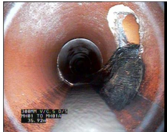
Photo: 13_13_170_A.jpg, 00:05:32 36m, Connection other than junction, at 3 o'clock, diameter 150mm
