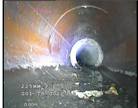
Photo: 3_3_35_A.jpg, 00:00:05 0m, Settled deposits, fine, 05% cross-sectional area loss
