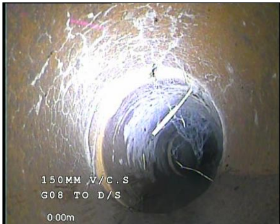
Photo: 8_8_85_A.jpg, 00:00:05 0.3m, Joint displaced, medium
