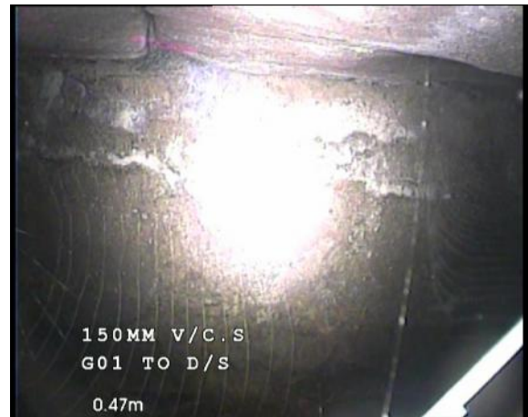
Photo: 1_1_33_A.jpg, 00:00:22 0.5m, Finish node type, other special chamber reference number: D/S Remarks: CONNECTION ONTO STONE CULVERT
