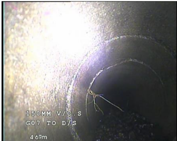
Photo: 7_7_79_A.jpg, 00:00:42 4.7m, Fracture, circumferential, from 9 to 3 o'clock
