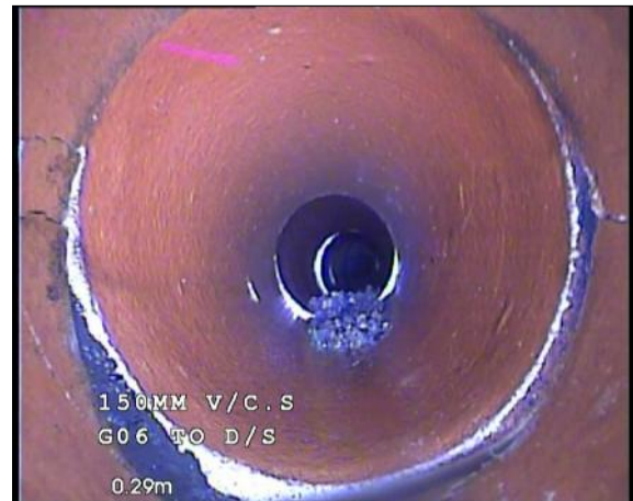
Photo: 6_6_64_A.jpg, 00:00:13 0.3m, Joint displaced, medium, Start
