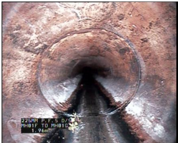
Photo: 29_29_310_A.jpg, 00:00:06 0m, Deformed sewer/drain, 10%, Start
