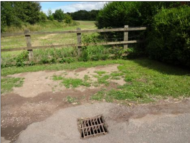
Photo: DSC02087.JPG 0m, General photograph taken at this point Remarks: LOCATION PHOTO
