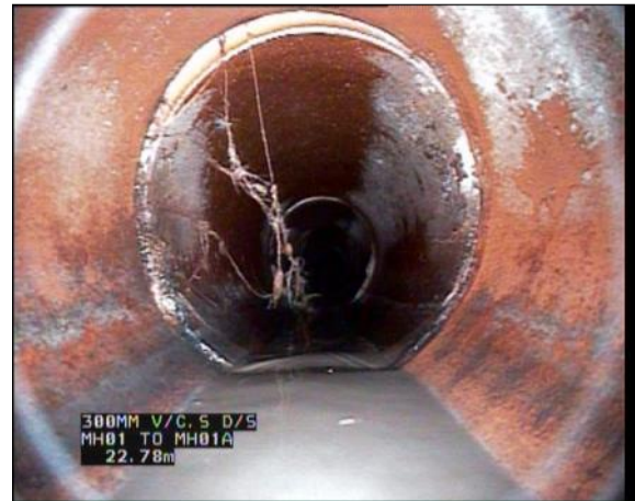
Photo: 13_13_166_A.jpg, 00:03:49 22.7m, Roots, fine at joint
