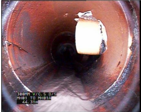
Photo: 13_13_177_A.jpg, 00:06:50 44.3m, Survey abandoned Remarks: OVERLAP COMPLETE TO INTRUDING CONNECTION
