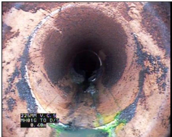
Photo: 33_33_369_A.jpg, 00:00:06 0.4m, Roots, fine at joint, Start
