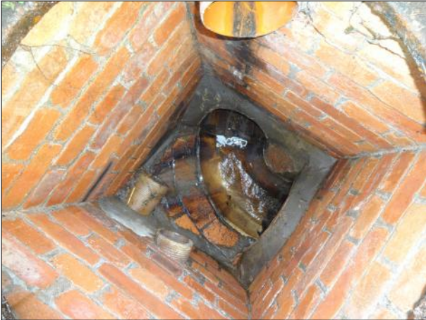
Photo: DSC02054.JPG 0m, Start node type, manhole, reference number : 01A
