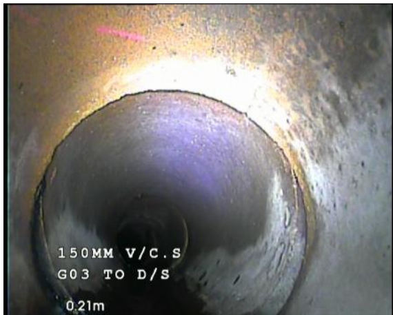
Photo: 4_4_44_A.jpg, 00:00:16 0.3m, Joint displaced, medium, Start
