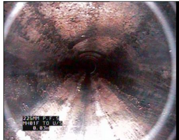
Photo: 32_32_341_A.jpg, 00:00:04 0m, Attached deposits, grease, from 7 to 5 o'clock, 5% cross-sectional area loss, Start Remarks: HEAVY FOUL POLLUTION THROUGHOUT
