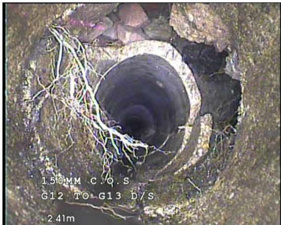
Photo: 16_16_219_A.jpg, 00:00:35 2.4m, Hole in drain/sewer, from 10 to 5 o'clock Remarks: LARGE HOLE
