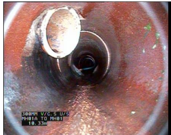
Photo: 11_11_103_A.jpg, 00:01:50 10.3m, Connection intruding, at 10 o'clock, diameter 150mm, intrusion 10%
