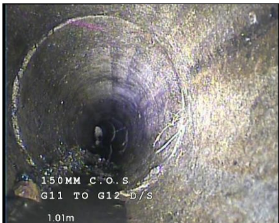
Photo: 15_15_212_A.jpg, 00:00:19 1m, Roots, fine at joint, Start
