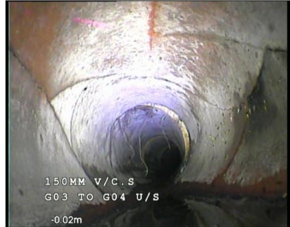
Photo: 5_5_52_A.jpg, 00:00:07 0m, Cracks, multiple, from 12 to 12 o'clock
