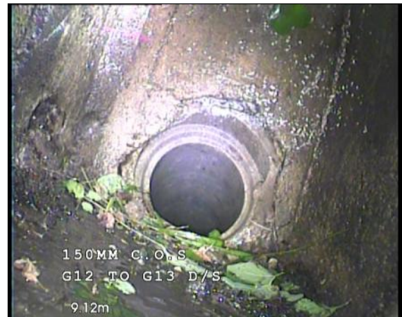
Photo: 16_16_225_A.jpg, 00:01:56 9.1m, Finish node type, gully reference number: G13 Remarks: GULLY 13
