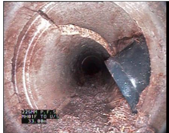
Photo: 32_32_362_A.jpg, 00:06:03 33m, Connection intruding, at 3 o'clock, diameter 150mm, intrusion 10%
