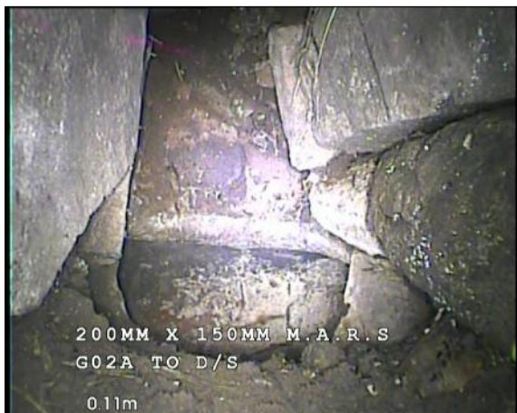
Photo: 30_30_320_A.jpg, 00:00:14 0m, Displaced bricks, from 7 to 5 o'clock
