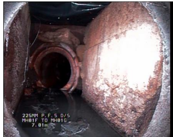
Photo: 29_29_313_A.jpg, 00:01:48 7.1m, Finish node type, manhole reference number: 01G Remarks: BURIED MH01G TRACED & EXPOSED
