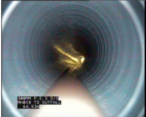
Photo: 25_25_284_A.jpg, 00:09:48 64.5m, Line deviates right Remarks: SLIGHT
