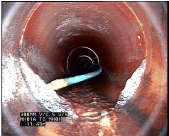
Photo: 11_11_106_A.jpg, 00:02:16 11.4m, Attached deposits, other, at 6 o'clock, 5% cross-sectional area loss, Start Remarks: DRAIN RODS (REMOVED AFTER SURVEY)
