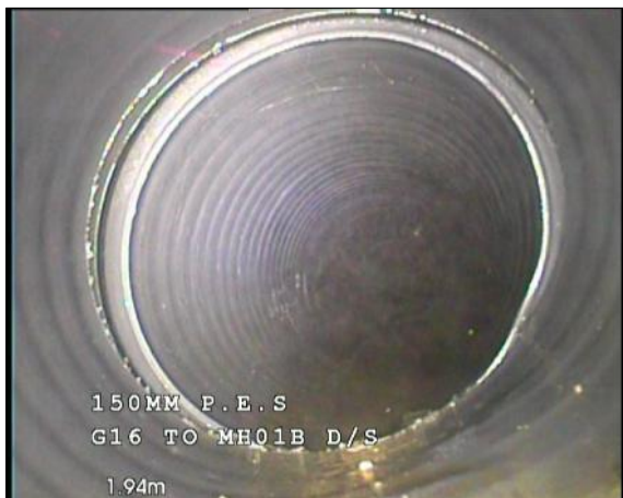
Photo: 19_19_235_A.jpg, 00:00:28 2m, Deformed sewer/drain, 05%
