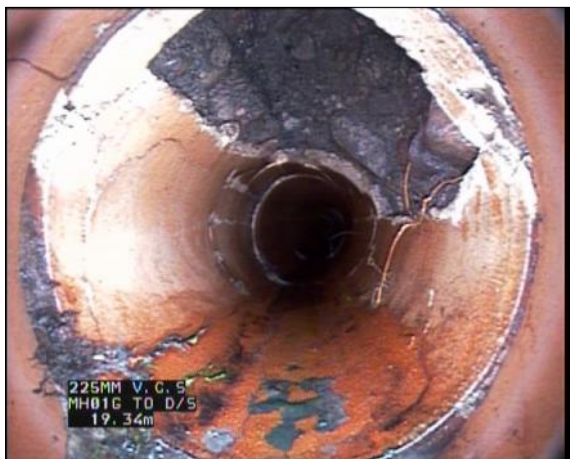
Photo: 33_33_379_A.jpg, 00:03:22 19.3m, Hole in drain/sewer, from 10 to 3 o'clock Remarks: LARGE HOLE
