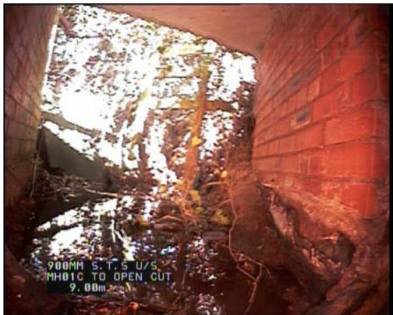
Photo: 28_28_302_A.jpg, 00:01:05 9m, Finish node type, other special chamber reference number: OPEN CUT Remarks: OPEN CUT DITCH
