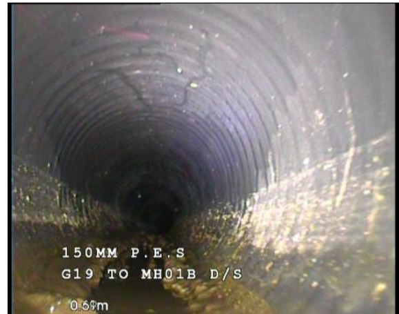
Photo: 21_21_240_A.jpg, 00:00:19 0.6m, Settled deposits, fine, 05% cross-sectional area loss
