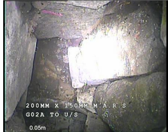
Photo: 31_31_332_A.jpg, 00:00:06 0m, Displaced bricks, from 7 to 5 o'clock
