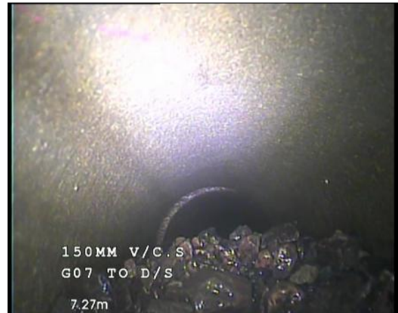
Photo: 7_7_82_A.jpg, 00:01:10 7.2m, Settled deposits, coarse, 70% cross-sectional area loss
