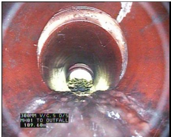
Photo: 12_12_149_A.jpg, 00:21:26 109.6m, Line deviates down
