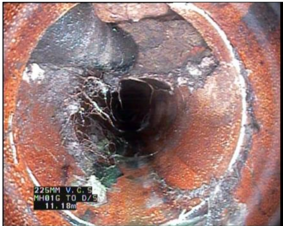
Photo: 33_33_375_A.jpg, 00:01:45 11.1m, Hole in drain/sewer, from 10 to 2 o'clock Remarks: LARGE HOLE
