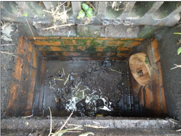
Photo: DSC02069.JPG 0m, Start node type, gully, reference number : G15 Remarks: GULLY 15
