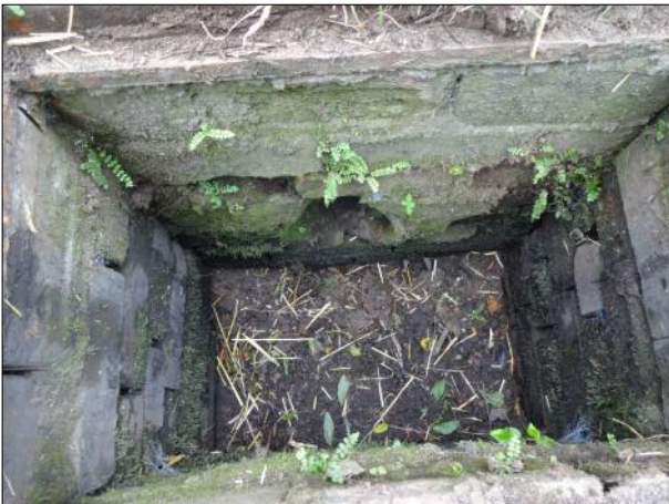
Photo: DSC02042.JPG 0m, Start node type, gully, reference number : G09 Remarks: GULLY 09
