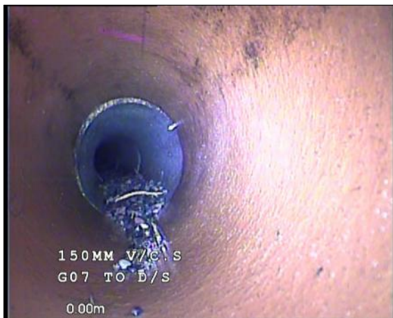
Photo: 7_7_15_A.jpg 0m, General remark Remarks: HEAVY DEBRIS REMOVED. GULLY OPERATING POORLY
