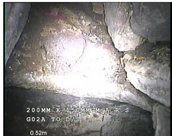
Photo: 30_30_322_A.jpg, 00:00:25 0.5m, Line deviates right Remarks: CONNECTION ONTO MAIN 225MM CARRIER
