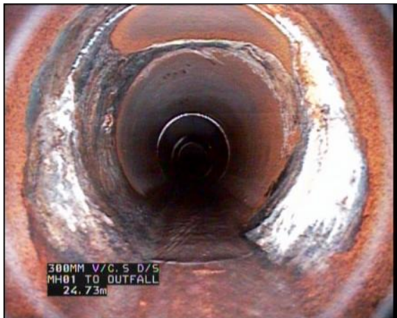
Photo: 12_12_122_A.jpg, 00:04:22 24.7m, Attached deposits, encrustation at joint, from 7 to 5 o'clock, 05% cross-sectional area loss
