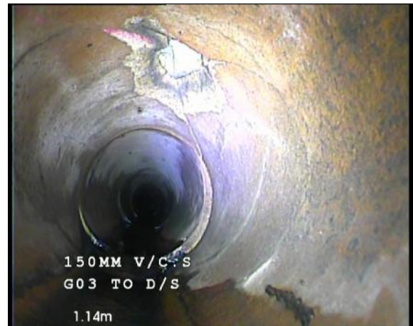
Photo: 4_4_47_A.jpg, 00:00:28 1.1m, Hole in drain/sewer, at 1 o'clock Remarks: SMALL HOLE
