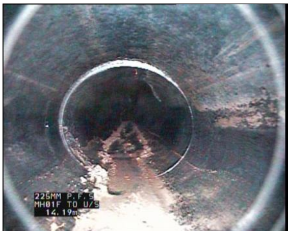
Photo: 32_32_346_A.jpg, 00:02:10 14m, Deformed sewer/drain, 10%, Start
