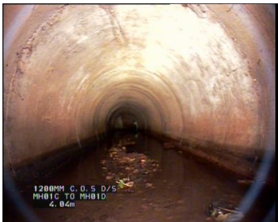
Photo: 26_26_288_A.jpg, 00:00:29 2.4m, Settled deposits, fine, 20% cross-sectional area loss, Start
