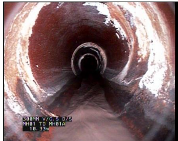
Photo: 13_13_158_A.jpg, 00:01:52 10.3m, Attached deposits, encrustation at joint, from 7 to 5 o'clock, 5% cross-sectional area loss, Start
