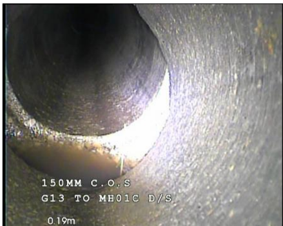
Photo: 22_22_244_A.jpg, 00:00:12 0.3m, Joint displaced, medium
