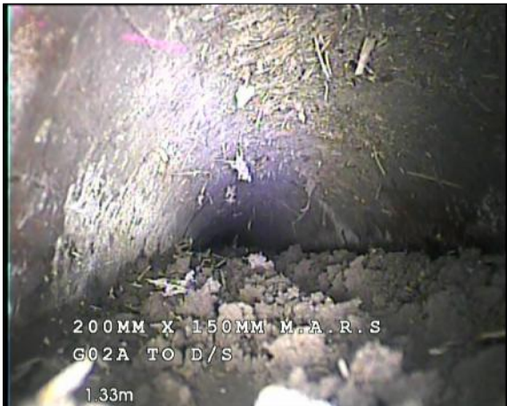
Photo: 30_30_327_A.jpg, 00:00:58 1m, Settled deposits, fine, 75% cross-sectional area loss Remarks: HEAVILY SILTED MAIN CARRIER
