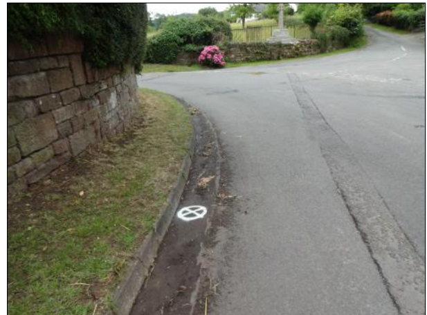
Photo: DSC02038.JPG, 00:01:07 4.6m, Survey abandoned Remarks: UNABLE TO CONTINUE. OBSTRUCTION TRACED & MARKED AT 10MTS 0.85MTS DEEP
