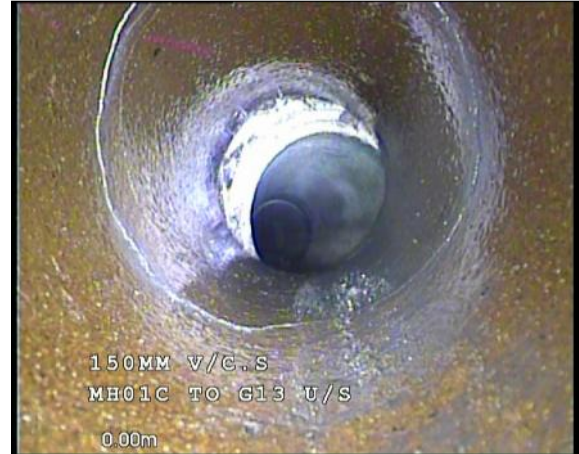
Photo: 24_24_272_A.jpg, 00:00:04 0.1m, Crack, circumferential, from 12 to 12 o'clock
