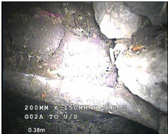
Photo: 31_31_334_A.jpg, 00:00:16 0.5m, Line deviates left Remarks: CONNECTION ONTO MAIN 225MM CARRIER
