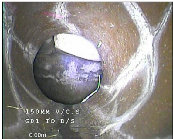
Photo: 1_1_32_A.jpg, 00:00:05 0m, Cracks, multiple, from 12 to 12 o'clock
