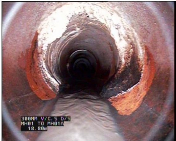
Photo: 13_13_162_A.jpg, 00:03:12 18.8m, Attached deposits, encrustation at joint, from 7 to 5 o'clock, 10% cross-sectional area loss
