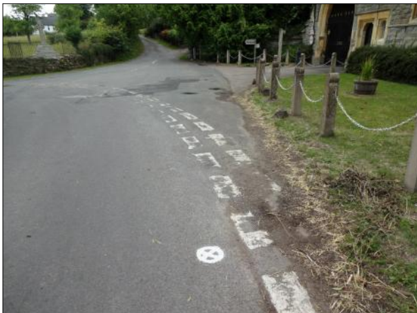
Photo: DSC02040.JPG, 00:01:10 7.2m, Survey abandoned Remarks: UNABLE TO CONTINUE. OBSTRUCTION TRACED & MARKED AT 19MTS 0.86MTS DEEP
