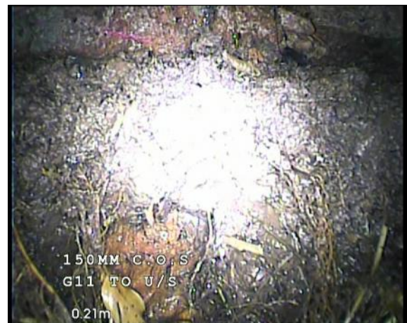
Photo: 14_14_208_A.jpg, 00:00:18 0.2m, Finish node type, other special chamber reference number: U/S Remarks: HEAD OF RUN
